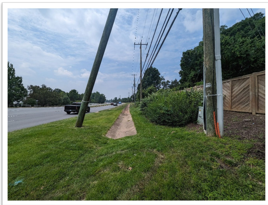
Field Photo 7: SB Cascades Pkwy looking south towards Oakbrook Court. Concrete ditch between Sta. 118+00 to Sta. 121+00.
